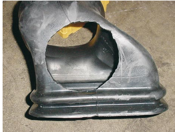
Figure 12 - Hole cut in duct transition
